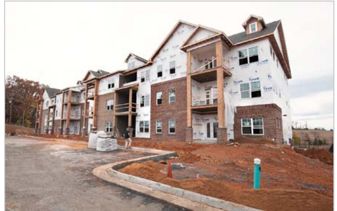
Apartment buildings are under construction at The Reserve at Stone Port in Rockingham County on Wednesday. Todd Dofflemyer, CEO of Charlottesville-based The Cathcart Group, said that if all goes well, the first tenants will be able to move into their new digs in December. (Photos by Michael Reilly / DN-R)
